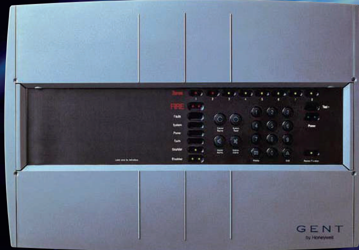
Xenex Control Panel
